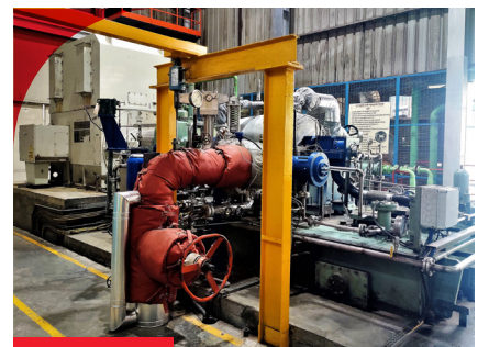
Biomass based turbine at Hapur
